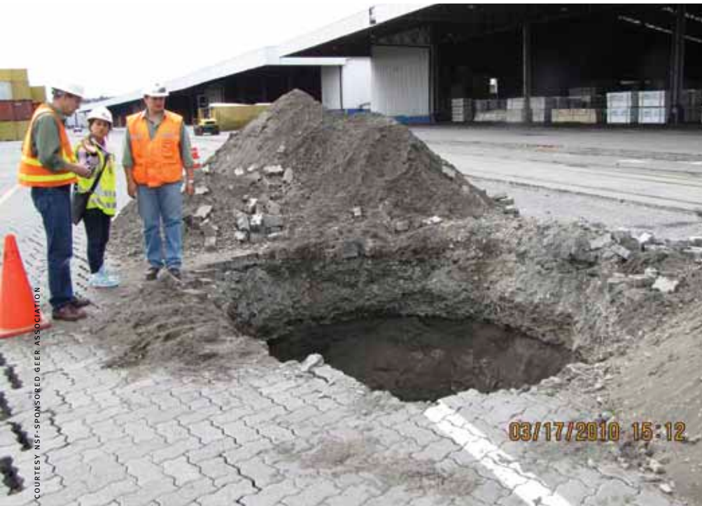
Members of the NSF-sponsored Geoengineering Extreme Events Reconnaissance Association (GEER) team, co-led by UC Berkeley professor Jonathan Bray (not pictured), inspect a sinkhole at the Port of Coronel in Chile, part of an international effort by engineers to understand effects of the 8.8 earthquake. "Most probably, the sinkhole was associated with the presence of drainage pipes where the material washed out when the sand layer liquefied," explains team member Dominic Assimaki, assistant professor of civil and environmental engineering at Georgia Tech, who photographed the damage.
